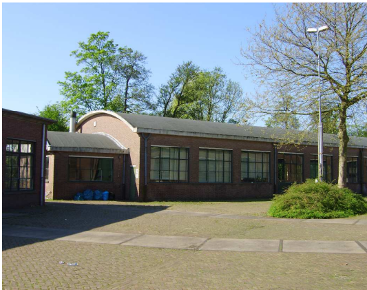
Fig. 11. Workshop roofed with barrel vault, formal military complex known as 'het Defensie-eiland' in Woerden, The Netherlands.
