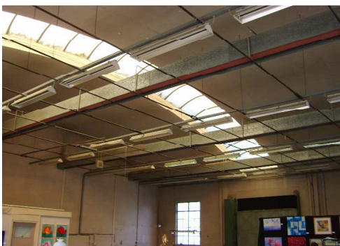
Fig. 8: The workshop of the former military complex 'het Defensie-eiland' in Woerden, the roof lights run parallel to the span.
